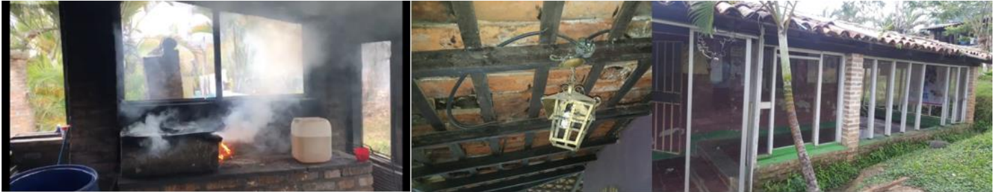
Figure 1. From right side, Kitchen facilities at Hogar CREA during a normal day of meal preparation. The wood burning stove on the campus, produces harmful emissions inside kitchen. In the middle, broken and unsafe light fixture in the classroom. On the left side, unsafe hanging electric wires from the roof with no exterior lighting system right where you need it.
