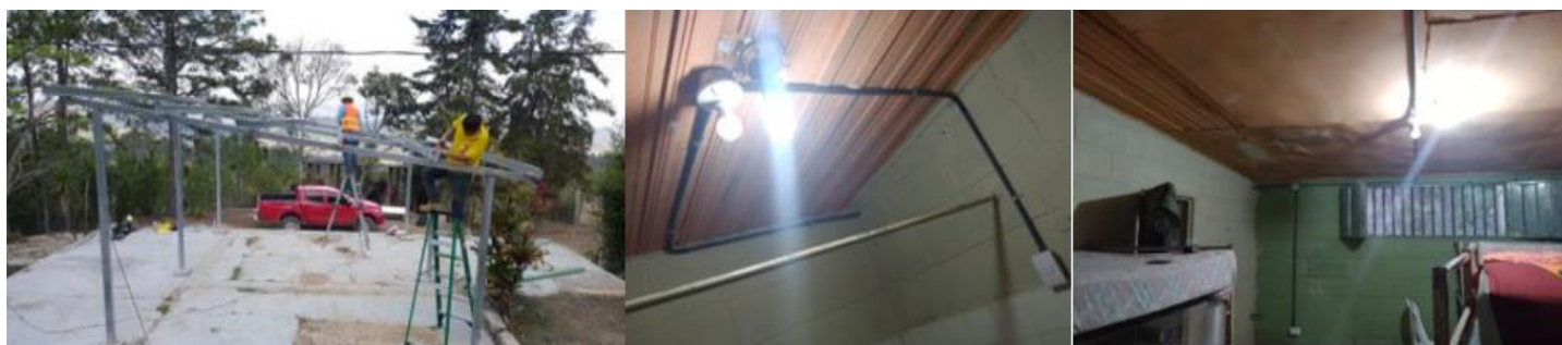
Figure 4. From left side, starting with new PV structure to hold solar panels in the system in phase one. In the middle and on the right side, new LED wiring, connections with insulation and new electric switches.
