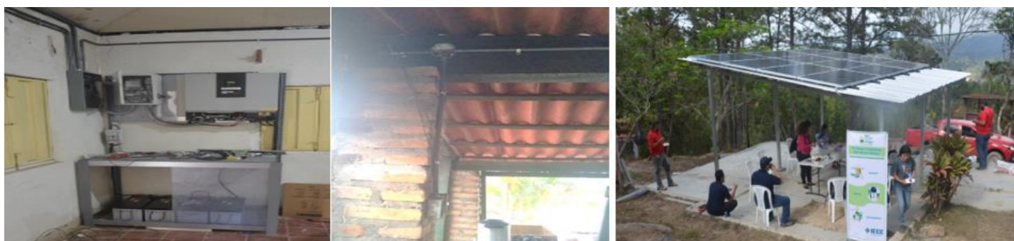
Figure 3. From left side, Controller Box and batteries in phase one. In the middle, new wiring, insulation and connections inside building. On the right side, a lunch break for a group of volunteers at Hogar CREA, technicians and local volunteers from IEEE Honduras section under the new PV structure that was built to install solar panels.
